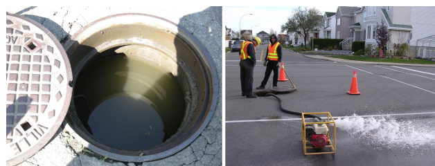
Figure 1. Flooded air-vacuum valve vault.
